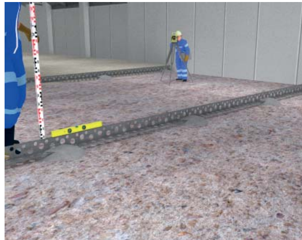
Adjusting UNIRAIL 40-60 for height using an optical sight level and measuring staff.
